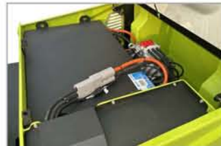
Crane hanging battery, easy to replace, with maximum capacity of 450Ah
